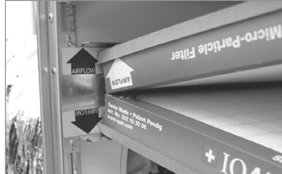
6. Ensure that you align the filters with the airflow arrows matching the airflow arrows on the cabinet.
